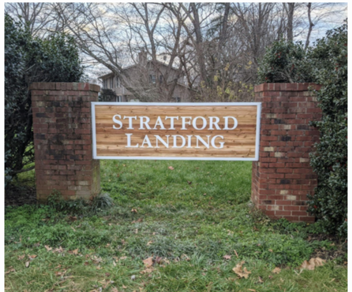
The brick pillars supporting the three new Stratford Landing entrance signs are in need of repair. Replacing the pillars would be infeasible with Fairfax County's new zoning laws.
